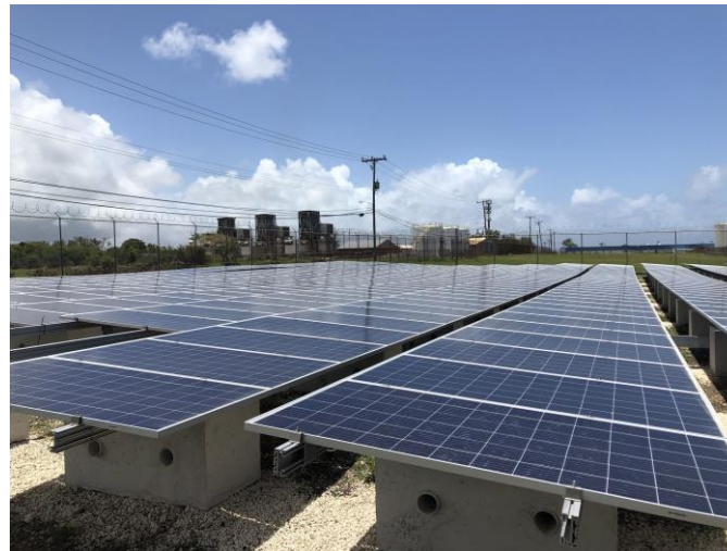
Solar PV system Barbados airport
